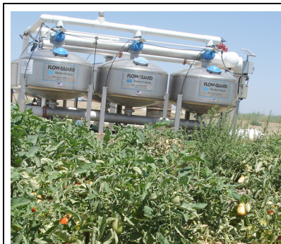
Filters are used to remove sand and other particles from water before flowing through drip irrigation lines stretched through a nearby field of processing tomatoes.
